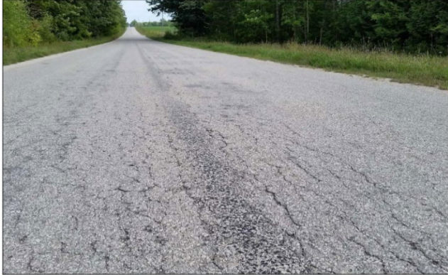
Alligator cracking throughout road
