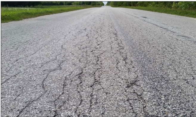
Alligator and map cracking
