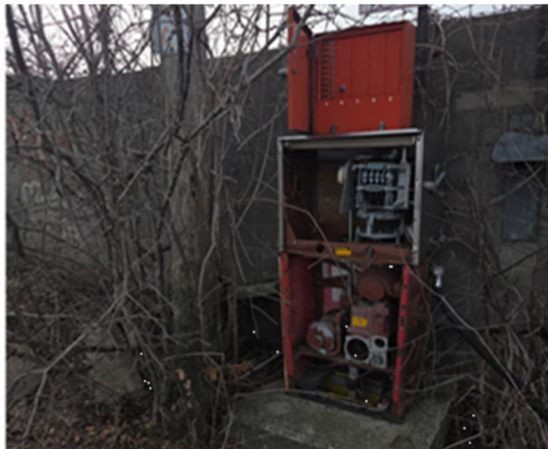
PHOTO 7: View of an abandoned fuel pump, located at the eastern portion of the Phase One Property, facing south.
