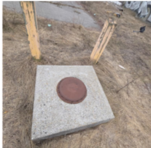
PHOTO 10: Additional view of the UST located on the east portion of the Phase One Property, facing west.
