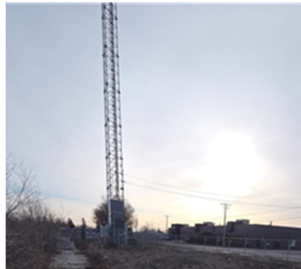
Photo 4: View of the communication tower and a transformer, near the central south limit of the Phase One Property, facing east.
