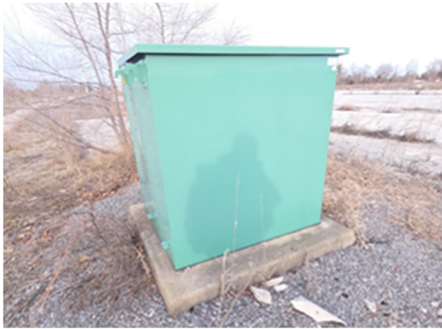
Photo 5: View of the transformer located near the central south limit of the Phase One Property, facing northwest.
