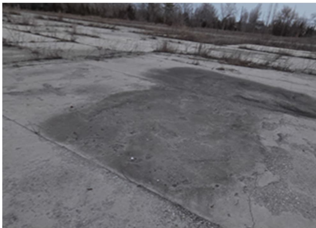
PHOTO 23: Additional staining within former building footprint, facing north.
