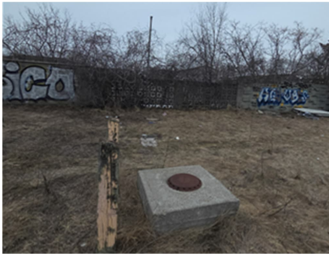
PHOTO 9: View of the UST and vent pipe located to the southeast of the abandoned fuel pump, located in the east portion of the Phase One Property, facing northeast.
