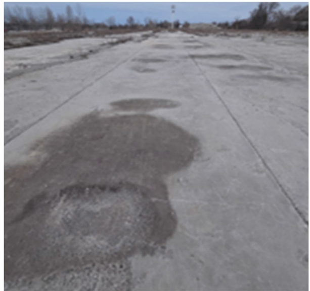
PHOTO 22: View of staining located near the central portion of the previous building footprint, facing west.
