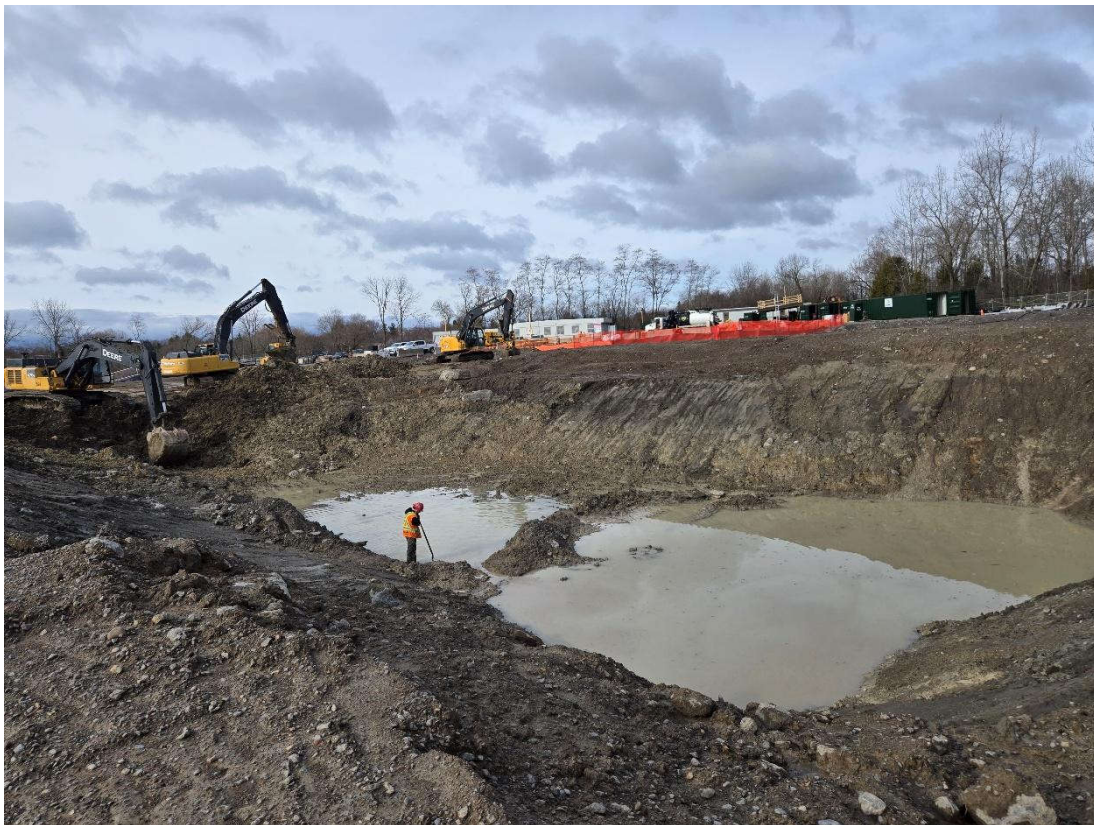
Photo 14: April 1 (aeration tanks)
