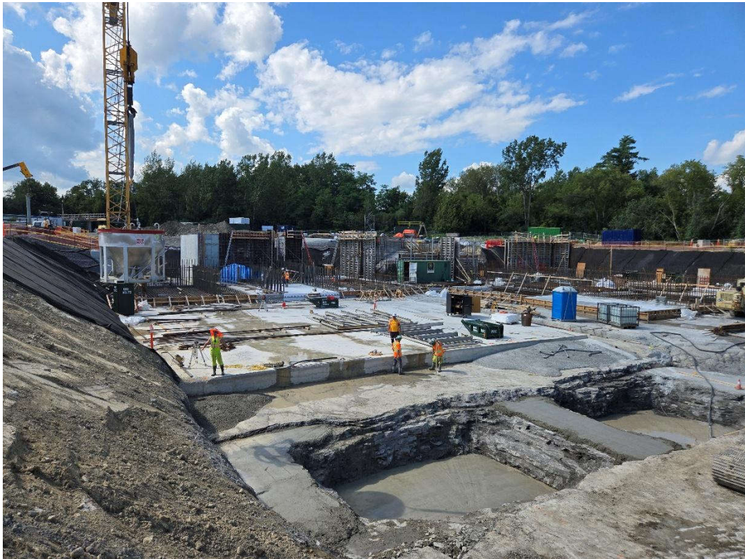
Photo 2: August 13 (aeration and clarifier tanks)
