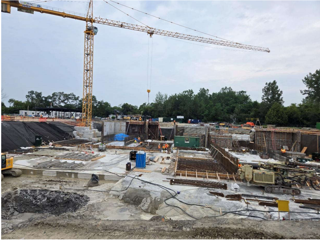
Photo 1: August 7 (aeration and clarifier tanks)
