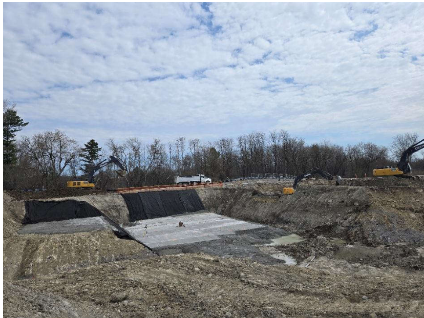
Photo 10: April 24 (aeration tanks)
