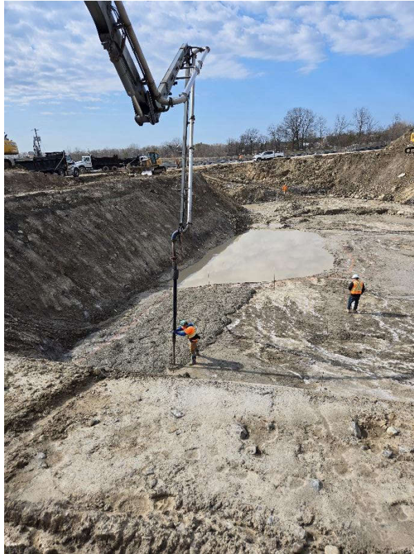
Photo 7: April 22 (aeration tanks)
