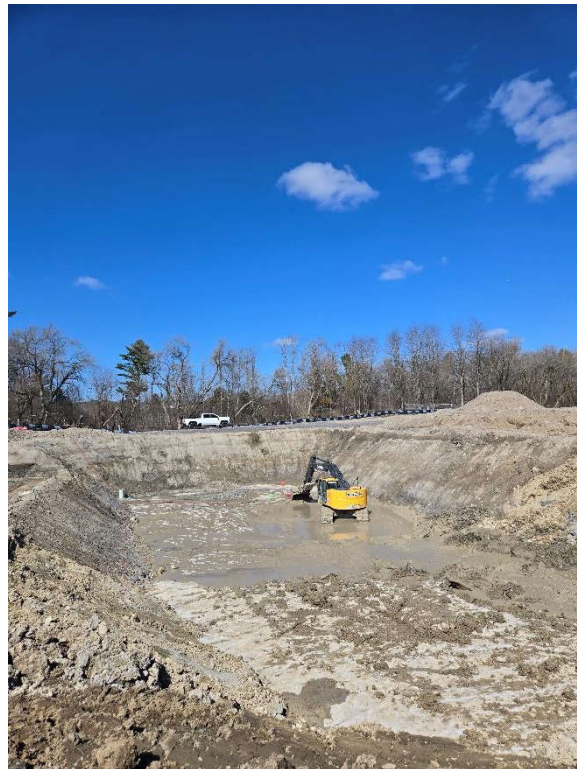
Photo 4: April 20 (aeration tanks)
