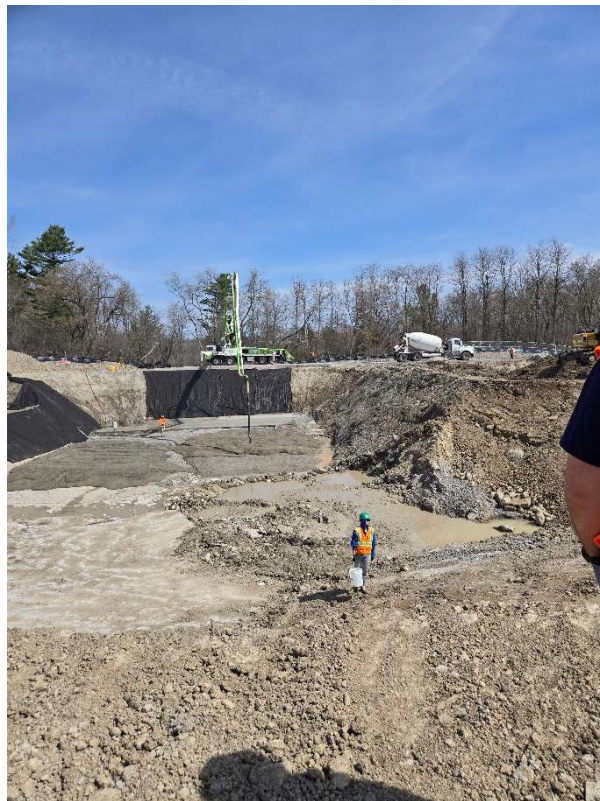
Photo 8: April 23 (aeration tanks)
