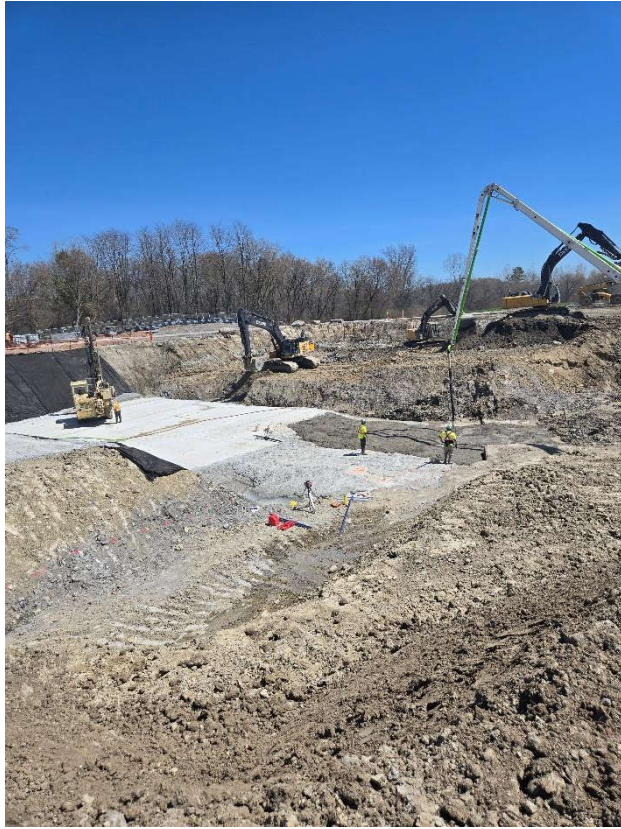
Photo 11: April 27 (aeration tanks)
