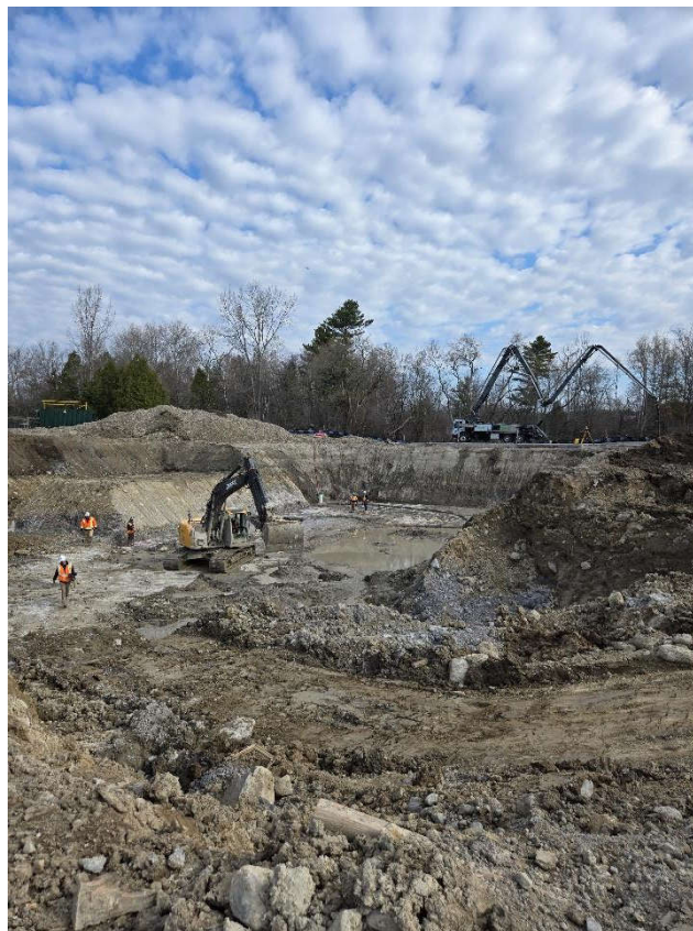
Photo 6: April 22 (aeration tanks)
