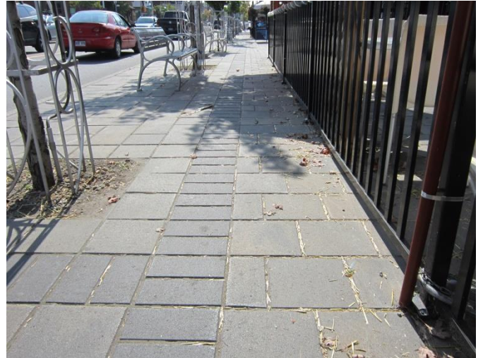
Not so Good = Tree pits with insufficient and loose fill materials are a hazard for everyone, particularly for elderly persons, persons with vision disabilities and persons using mobility aids
