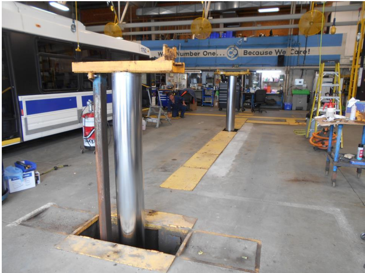
Photo of Existing Two Post Hoist System to be Replaced
