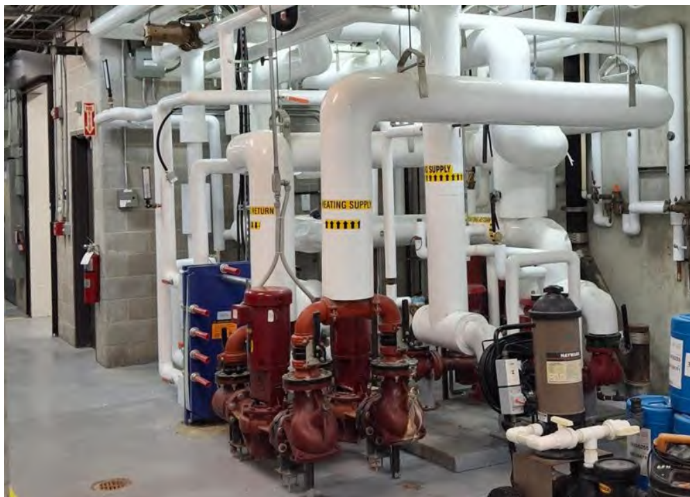
Heat exchanger and circulation pumps at Aquatic Centre
