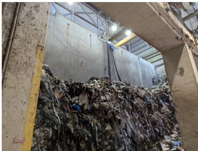
Photo 36: View of waste bunker within Tipping Building.
