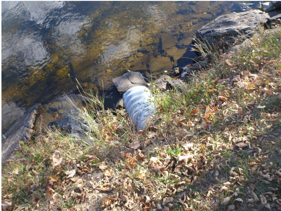
Photo 10: Outlet pipe, located on Madawaska street approximately 265 m west of Lanark Road, dischrnging stormwater south to the Madawaska River
