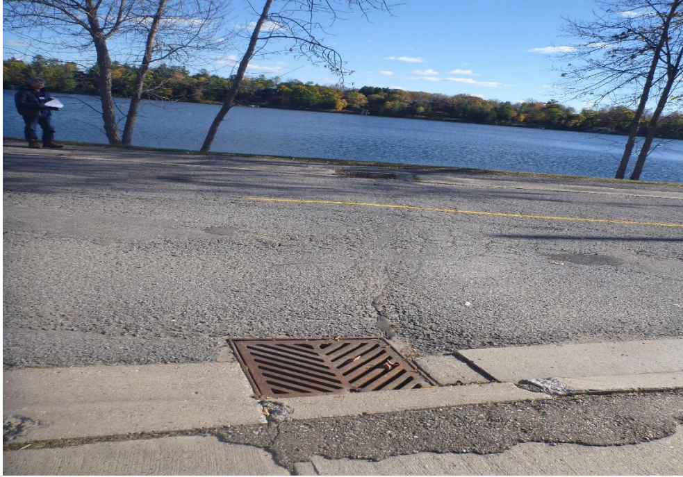
Photo 9: Drainage system, located on Madawaska Street approximately 265 m west of Lanark Road, conveying stormwater south to the Madawaska River
