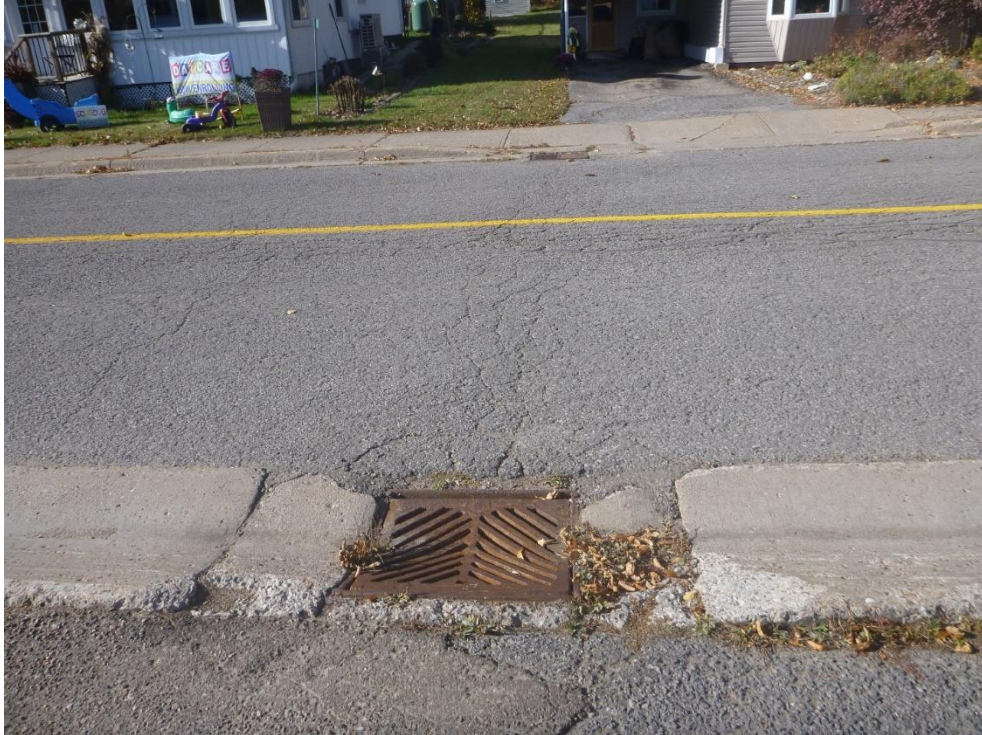
Photo 11: Drainage system, located on Gladstone street approximately 400 m west of Lanark Road, conveying stormwater south to the Madawaska River
