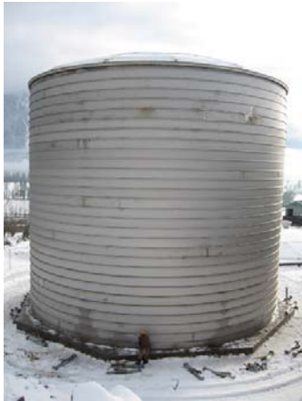
Water System Reservoir
