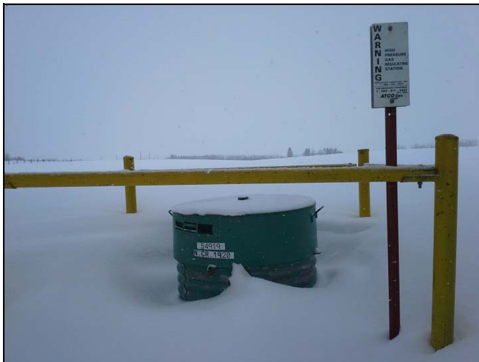
Photograph 6: Showing the high pressure gas regulating system located north of the acreage roadway (March 26, 2014).
