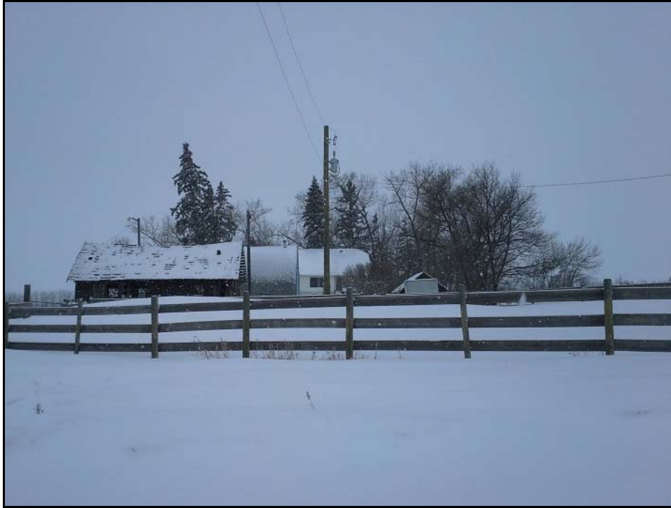
Photograph 15: Showing overhead power and an electrical transformer on the east portion of the acreage (March 26, 2014).
