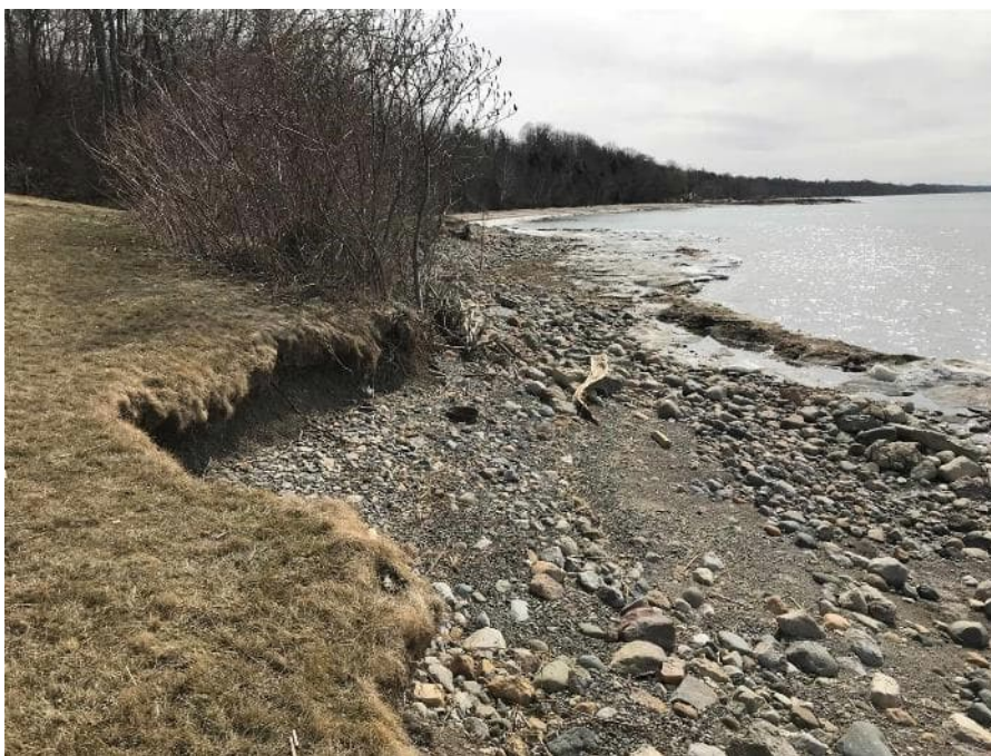
Photograph 24: Active erosion within grassy area west of the toe of slope near north end of property looking south on March 23, 2021.
