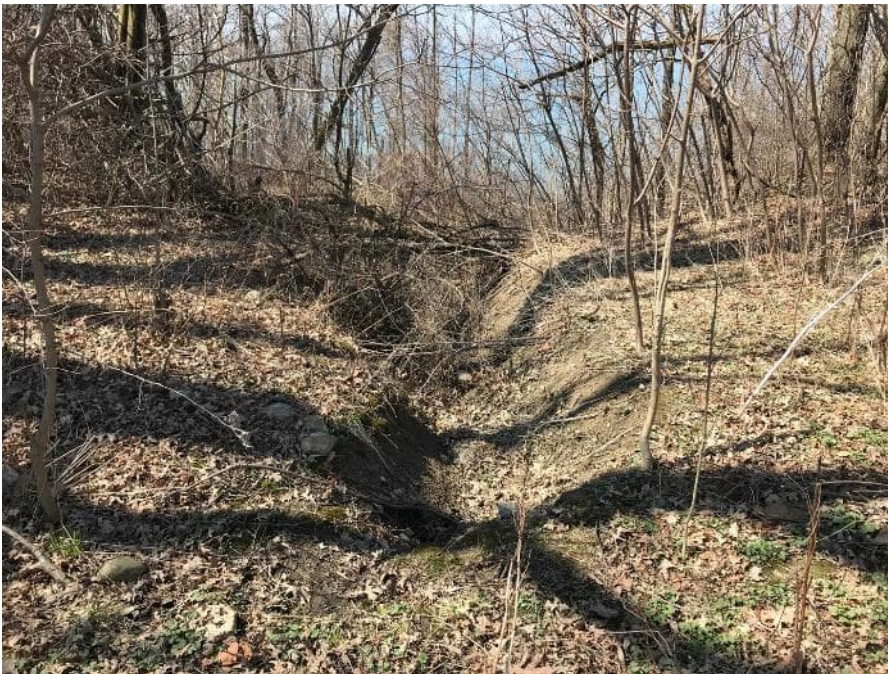
Photograph 23b: Gully at north end of site looking west. Gully caused by seepage from farm field drain pipe at top of slope on April 8, 2020.
