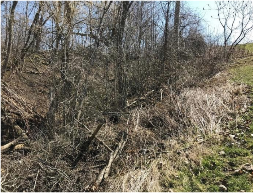
Photograph 17: Large erosion gully at south property line looking upslope on April 8, 2020. Gully caused by surface flows from north ditch along Cedar Point Line.
