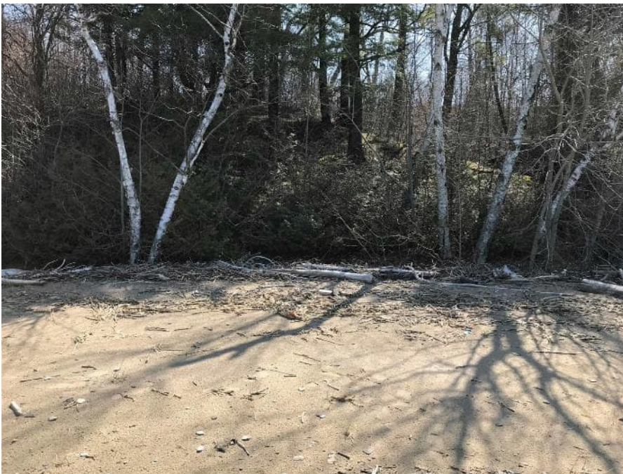
Photograph 3b: Section A-A' at beach looking upslope. No toe erosion on April 8, 2020; however, recent higher water levels have moved driftwood and debris landward compared to April 18, 2018 condition above.
