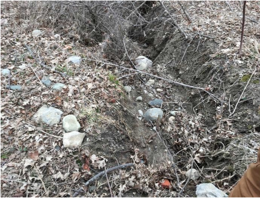
Photograph 23a: Gully at north end of site looking west. Gully caused by seepage from farm field drain pipe at top of slope on April 18, 2018.
