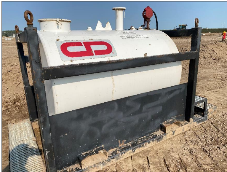
Photo 12 – Portable AST in the southwest-central portion of the Site.
