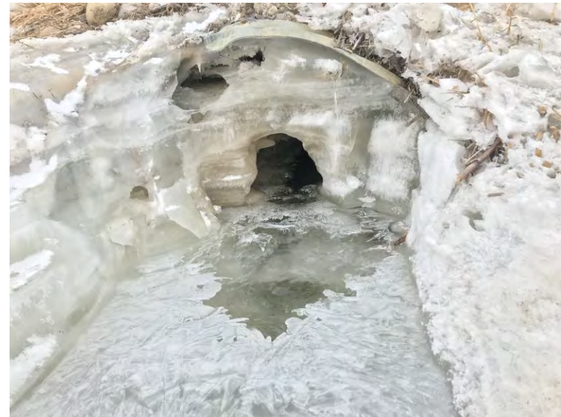
Frozen culvert following use of steaming equipment.
