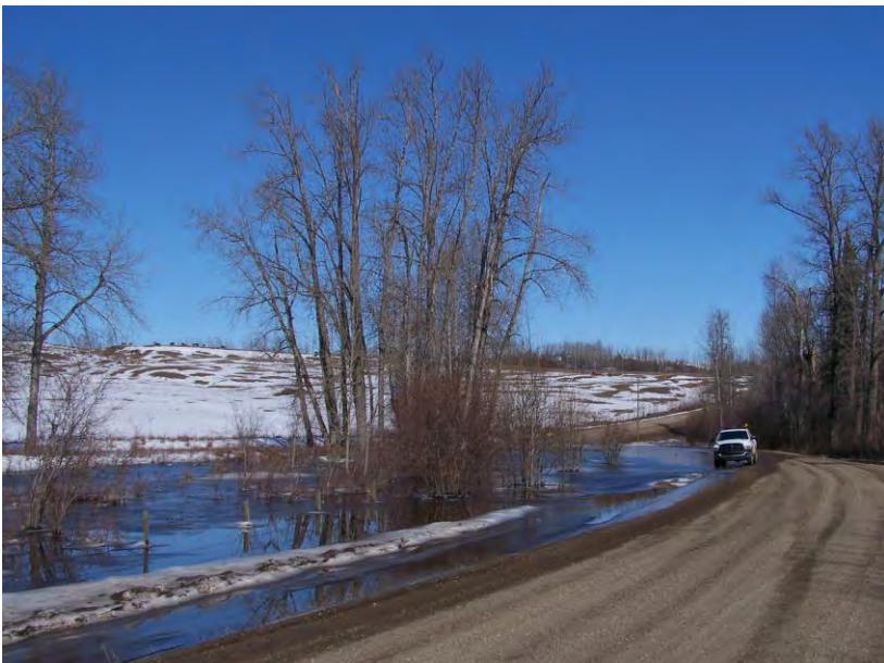
Spring runoff encroaching on rural roadway
