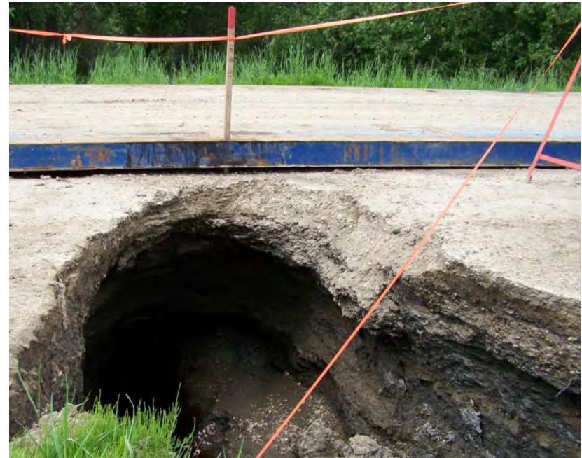
Washed out culvert on Range Road 63
