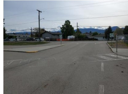
Figure 36. Faded markings within school site and driveway
