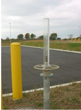
Valve in Storm (clean) Water Mode
