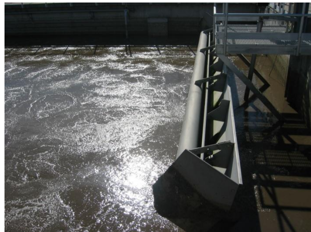
Photograph 2 ↑ SBR Decant Arm
