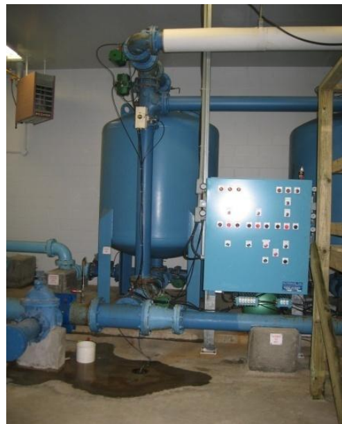
Figure 1-13: NHWTP Filter Photo
