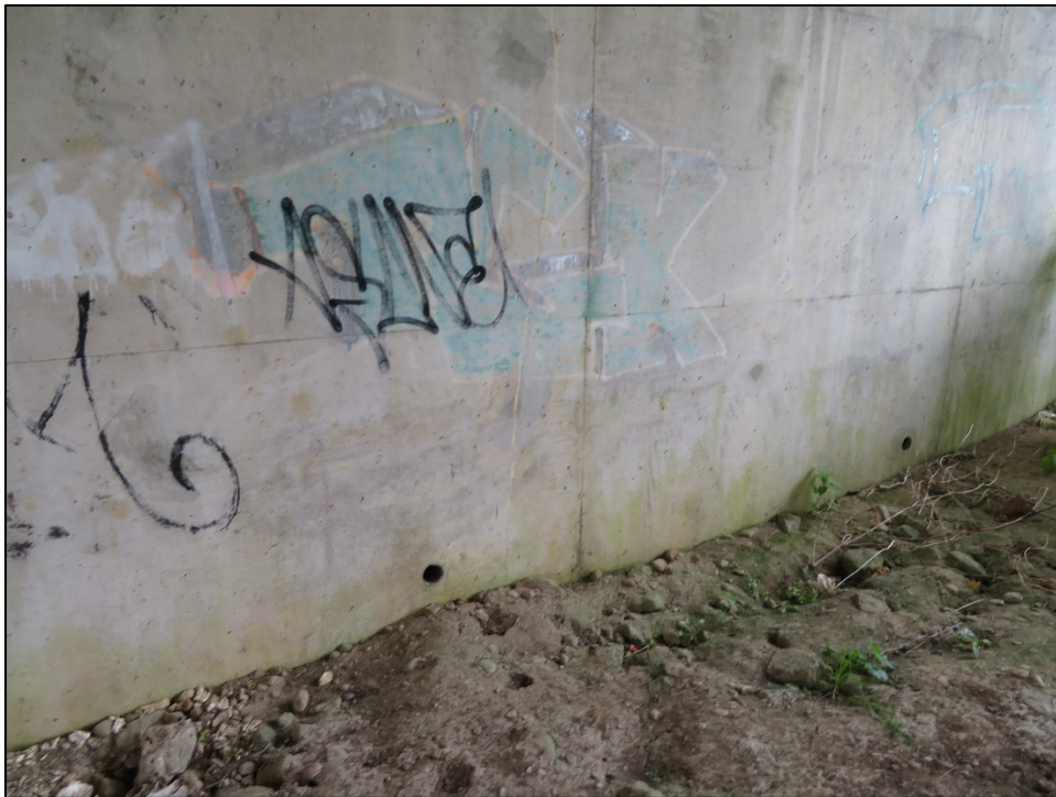
Photo P24 – Typical Condition of East Abutment (fair-to-good condition – cracking)
