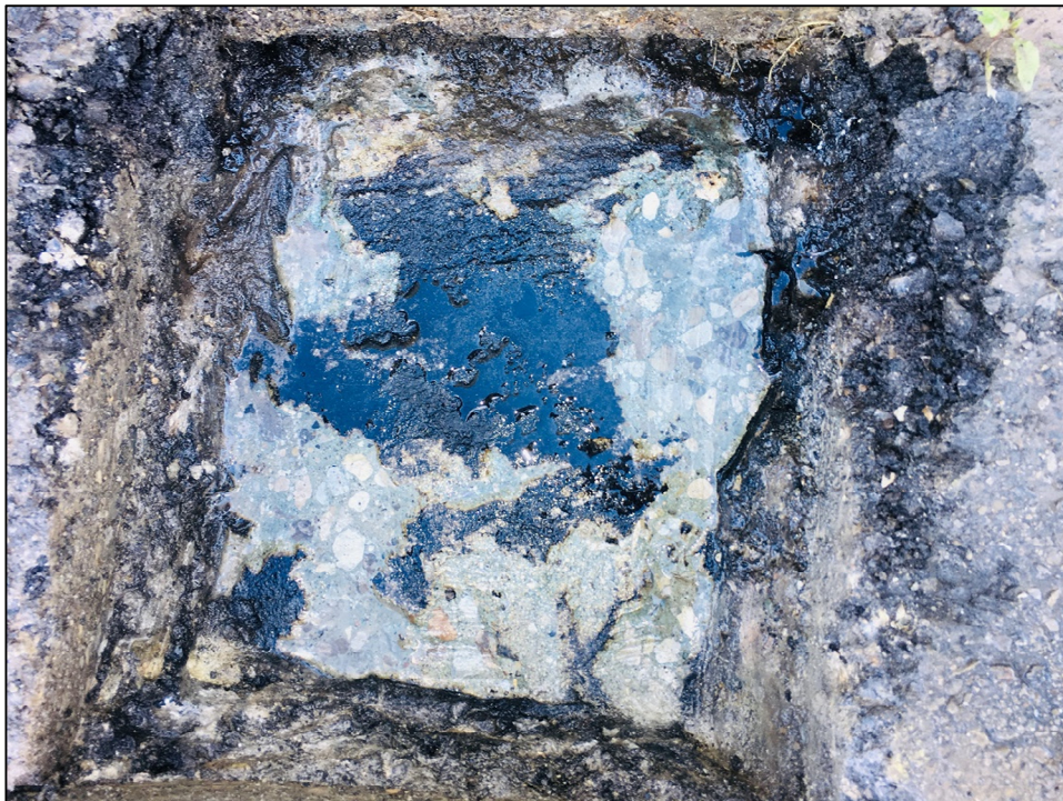
PHOTO S10 – SAWN SAMPLE S S10
