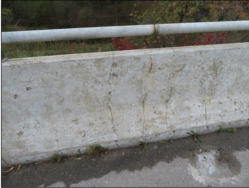
Photo P21 – Typical Condition of South Barrier Wall (fair-to-good condition – cracking and spalls)
