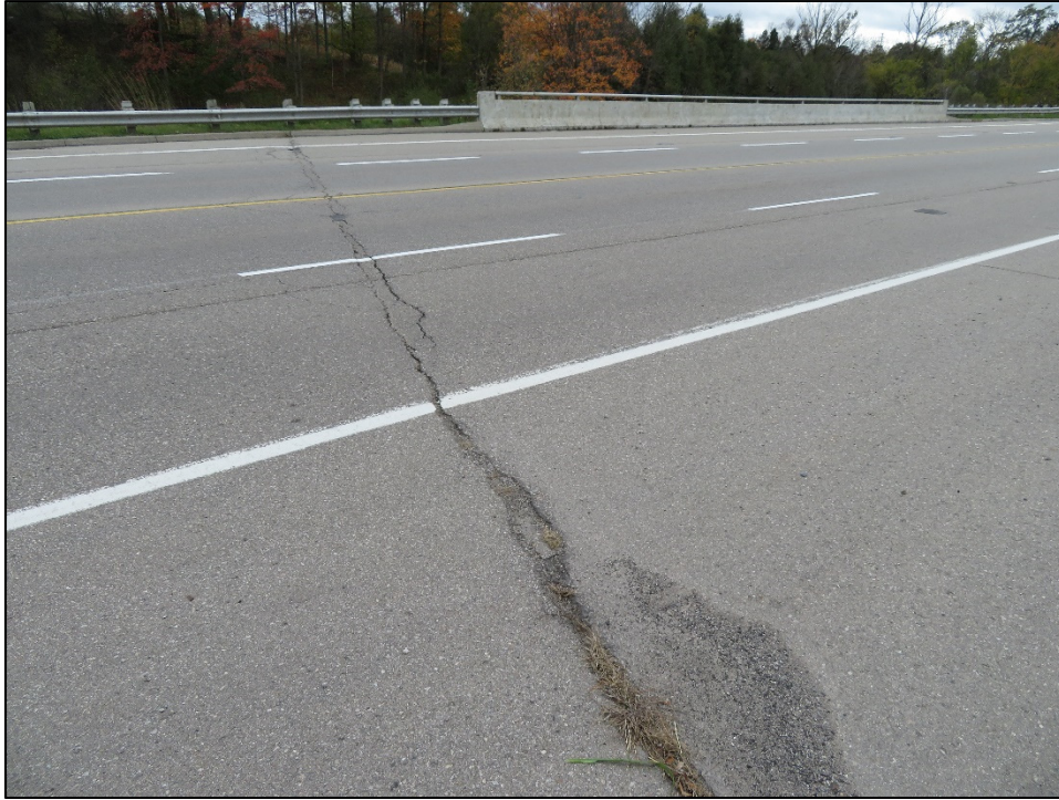
Photo P11 – Typical Condition of East Approach (fair condition – unsealed cracking)
