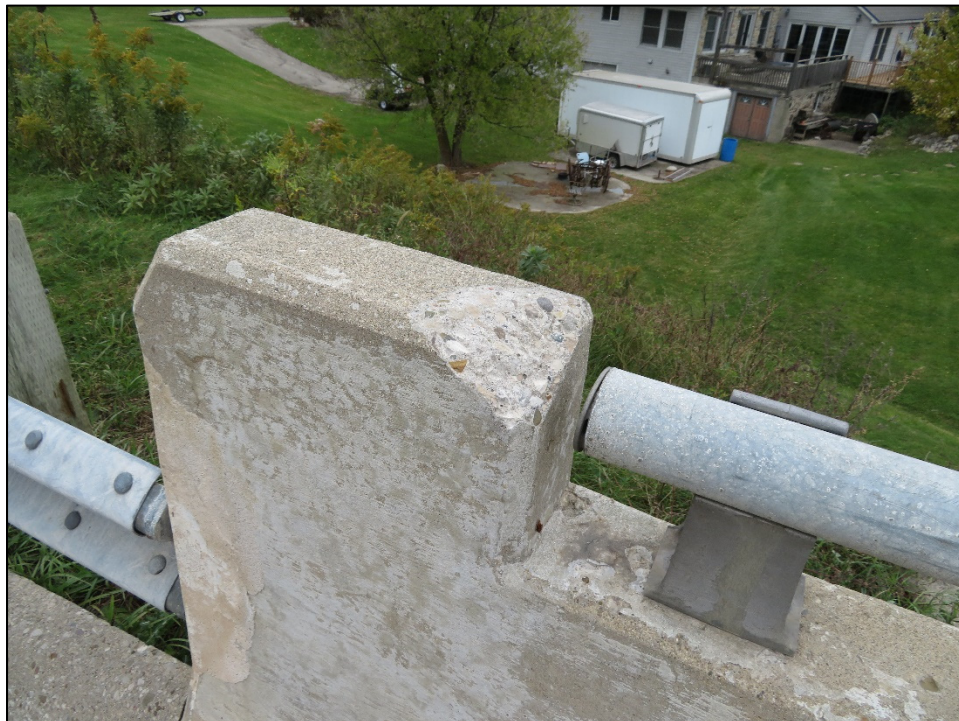
Photo P18 – Typical Condition of North Barrier Wall (fair-to-good condition – cracking, spalls and patch)
