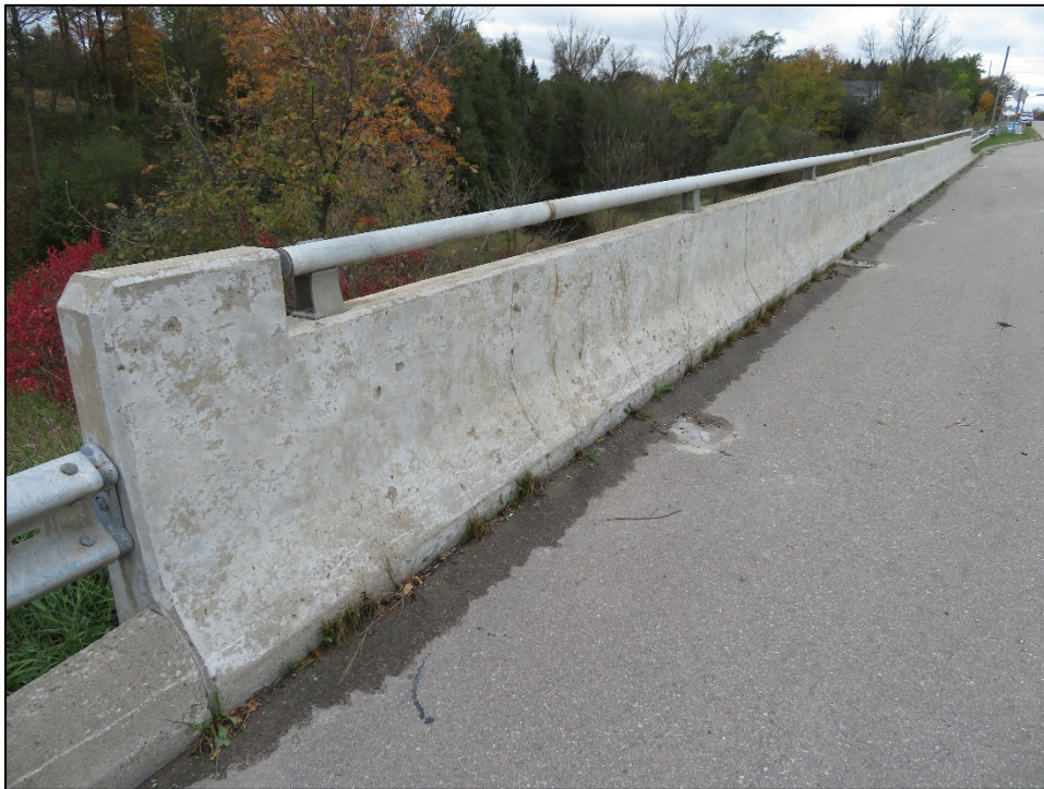
Photo P20 – Typical Condition of South Barrier Wall (fair-to-good condition – cracking and spalls)
