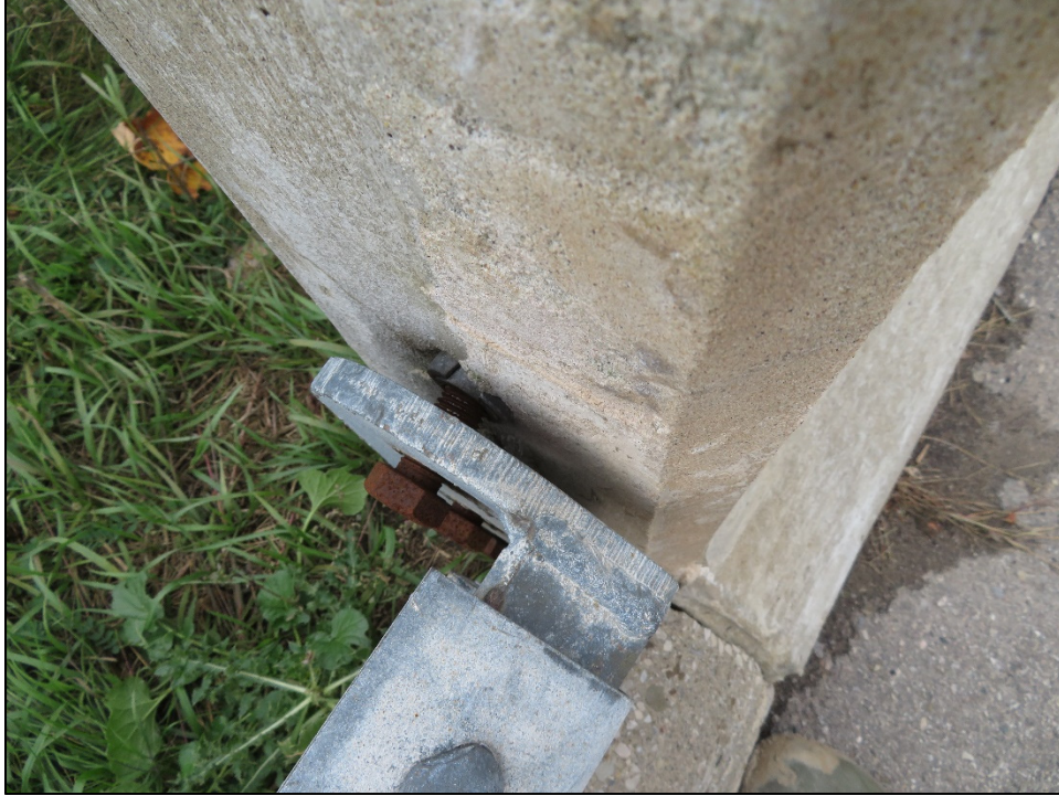
Photo P41 – Typical Condition of North-West Guiderail (connection to end post is separating)
