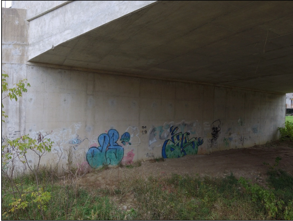
Photo P23 – Typical Condition of East Abutment (fair-to-good condition – cracking)
