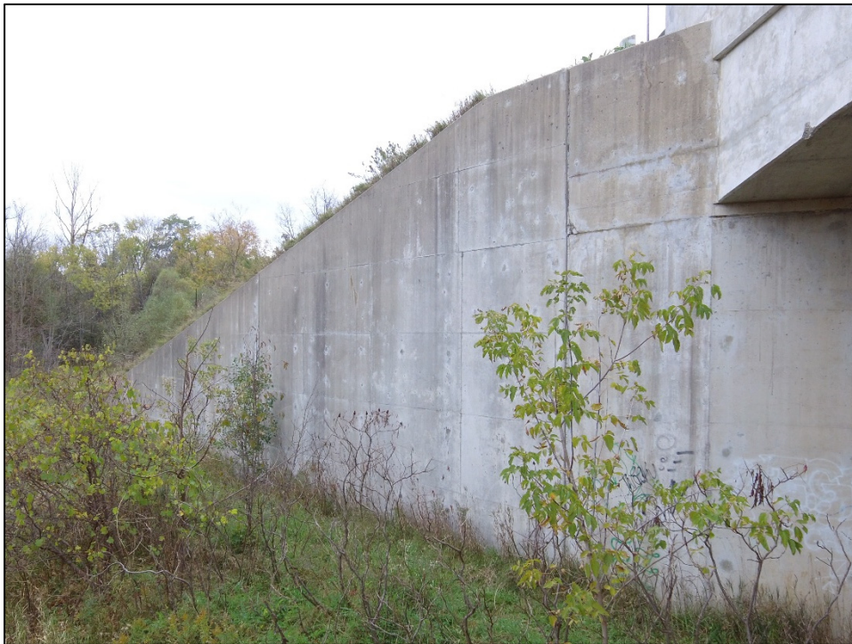
Photo P32 – Typical Condition of South-West Retaining Wall (fair condition – cracking)
