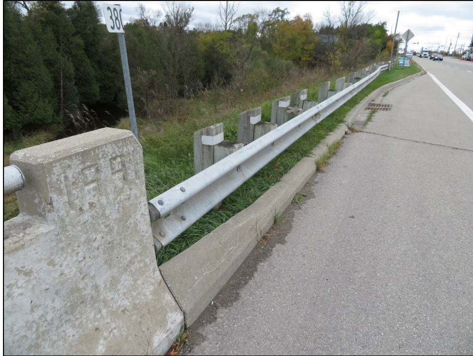
Photo P39 – Typical Condition of South-West Guiderail (connection to end post is separating)
