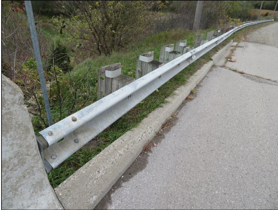
Photo P43 – Typical Condition of North-East Guiderail (connection to end post is separating)
