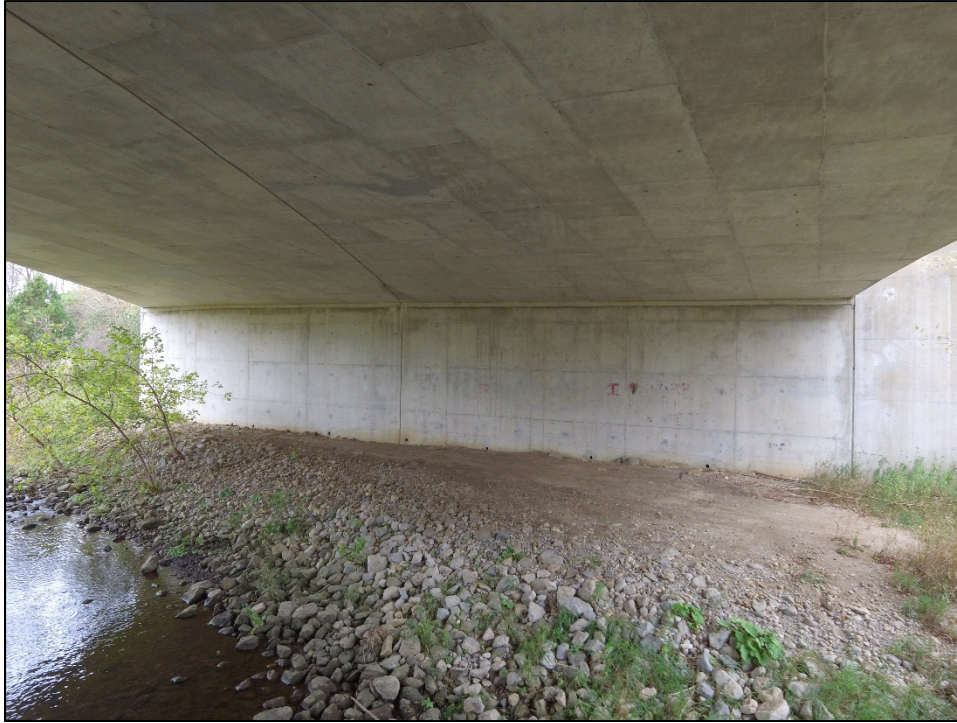
Photo P25 – Typical Condition of West Abutment (fair-to-good condition – cracking)
