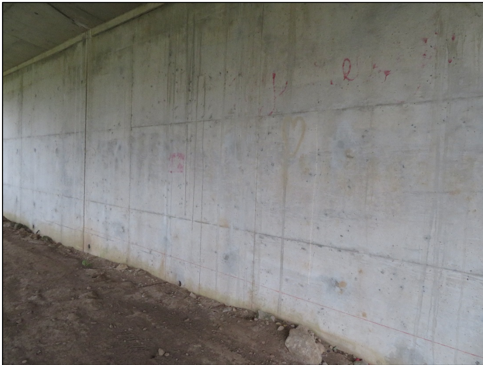
Photo P26 – Typical Condition of West Abutment (fair-to-good condition – cracking)
