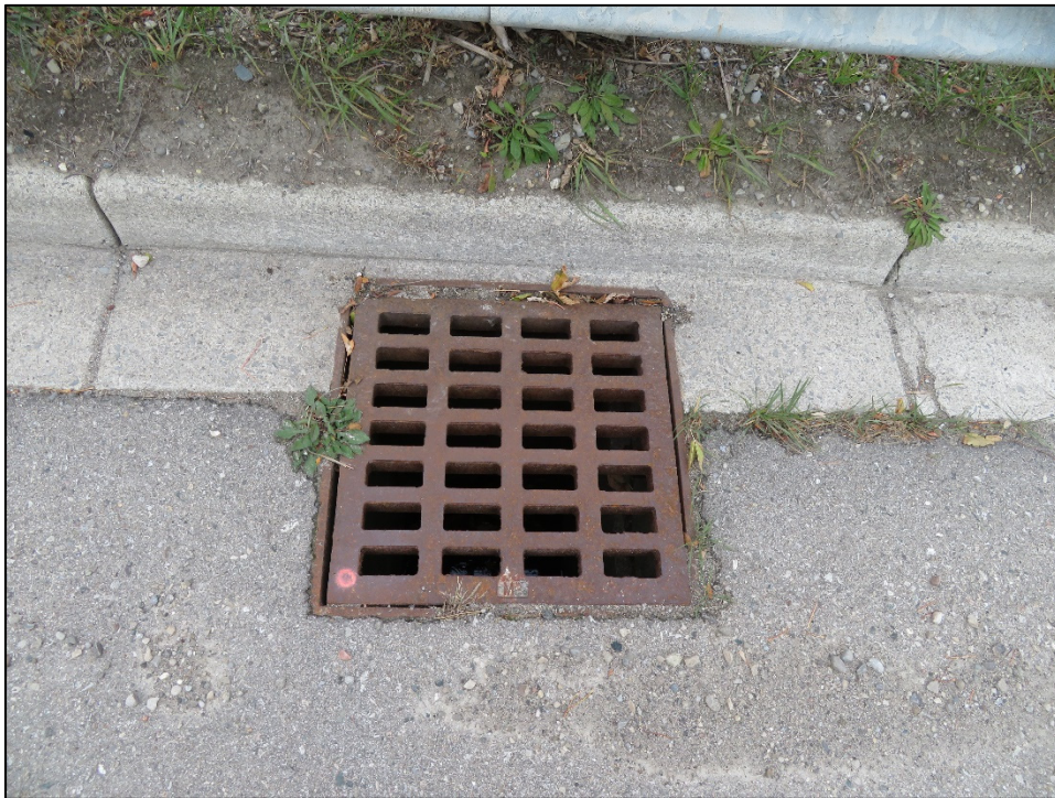
Photo P36 – Typical Condition of North-East Catchbasin
