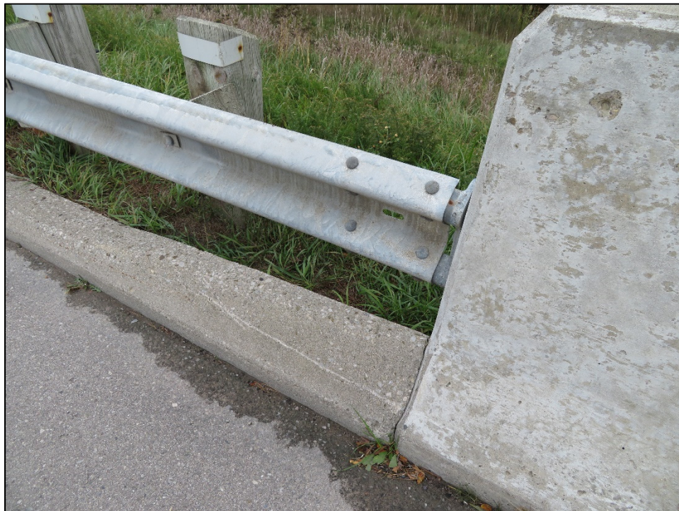
Photo P40 – Typical Condition of South-East Guiderail (connection to end post is separating)
