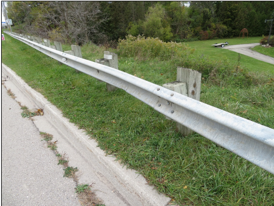
Photo P42 – Typical Condition of North-West Guiderail (minor impact damage)
