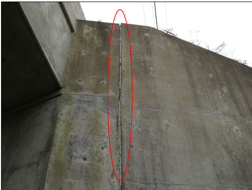
Photo P30 – Typical Condition of North-West Retaining Wall (fair condition - movement)
