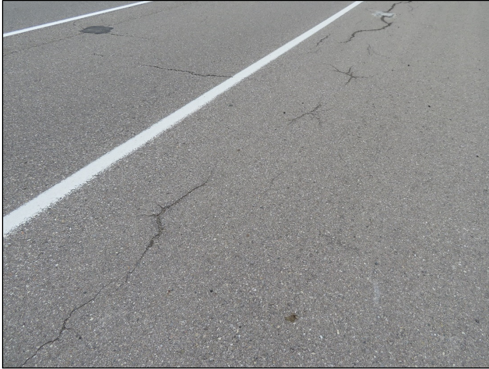
Photo P9 – Typical Condition of Asphalt Riding Surface (fair condition – unsealed cracking)
