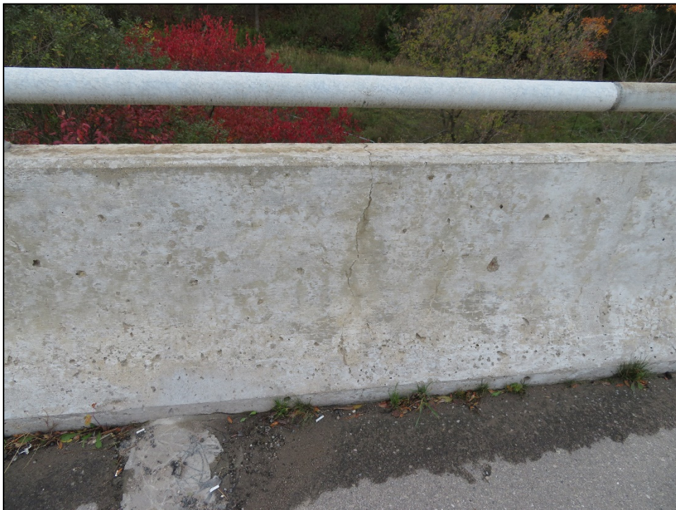
Photo P22 – Typical Condition of South Barrier Wall (fair-to-good condition – cracking and spalls)
