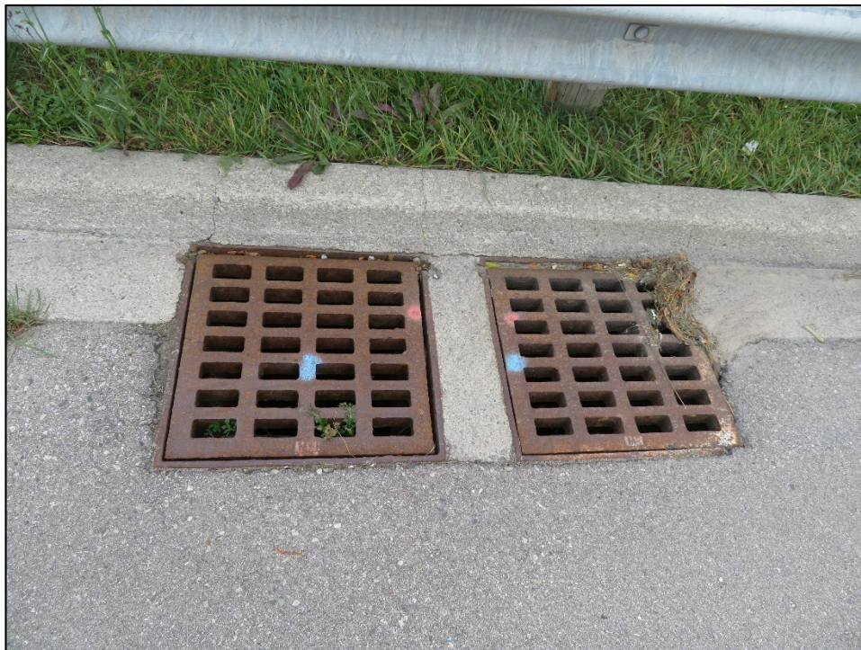
Typical Condition of Catchbasin @ South-West
