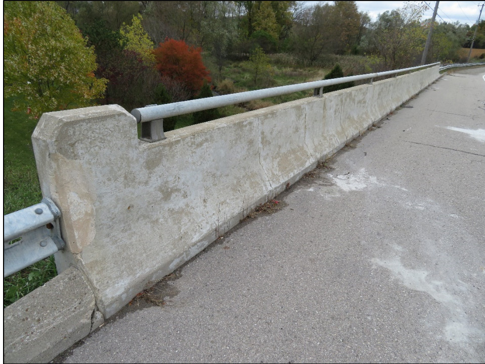
Photo P17 – Typical Condition of North Barrier Wall (fair-to-good condition – cracking, spalls and patch)
