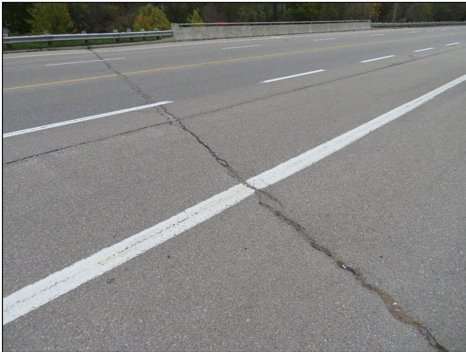
Photo P12 – Typical Condition of West Approach (fair condition – unsealed cracking)
