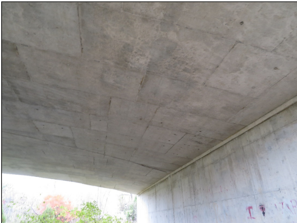
Photo P16 – Typical Condition of Soffit @ South-East (fair-to-good condition – wet areas and efflorescence staining at construction joint)
