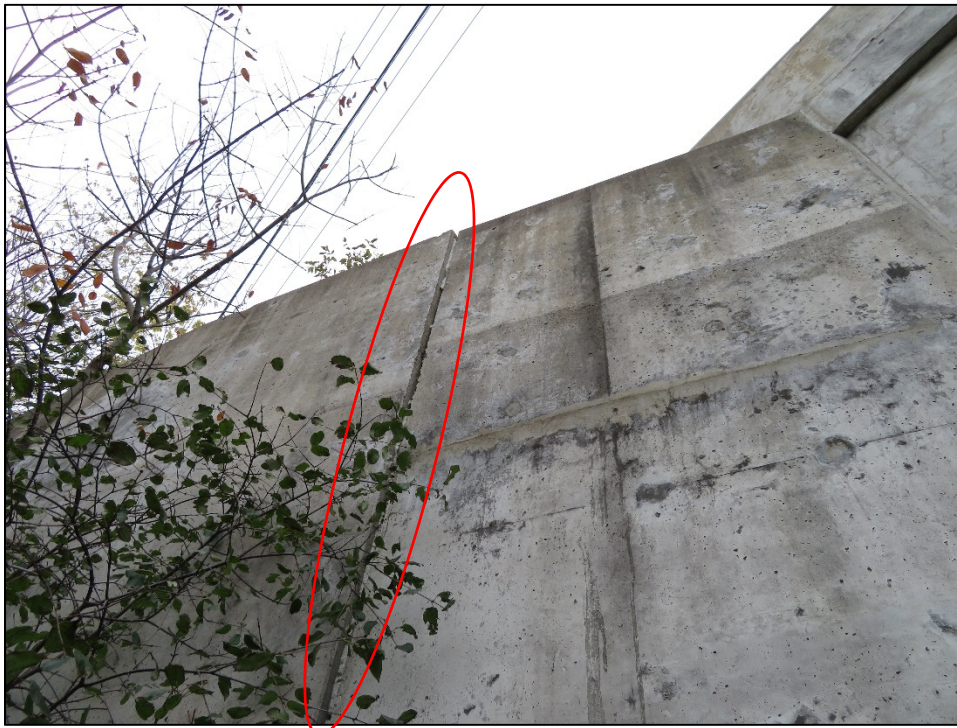
Photo P28 – Typical Condition of North-East Retaining Wall (fair condition - movement)
