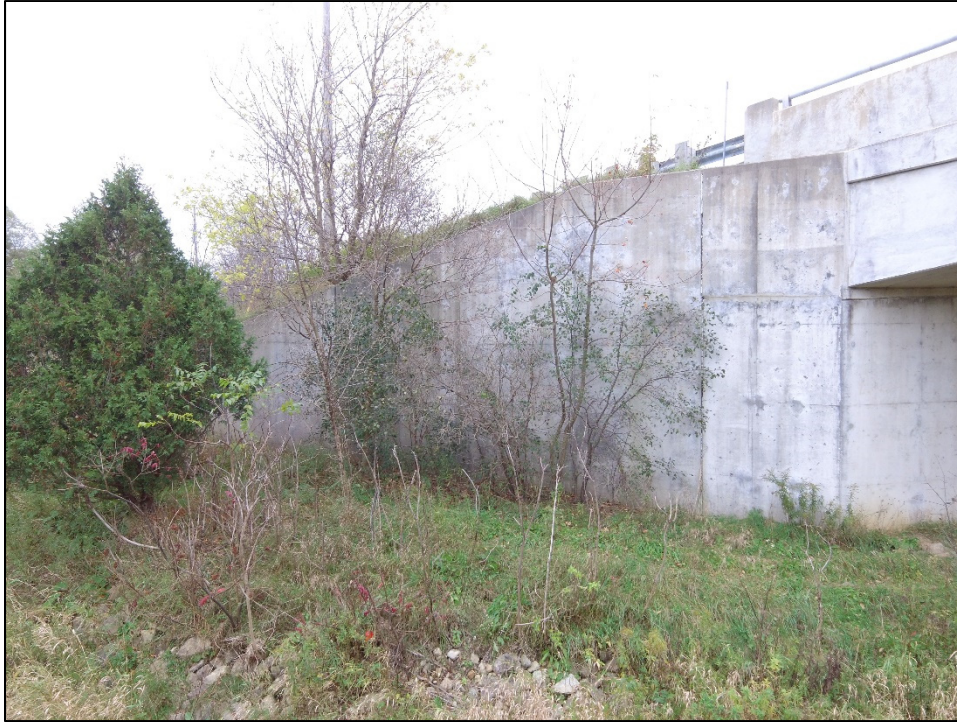
Photo P27 – Typical Condition of North-East Retaining Wall (fair condition - cracking)
