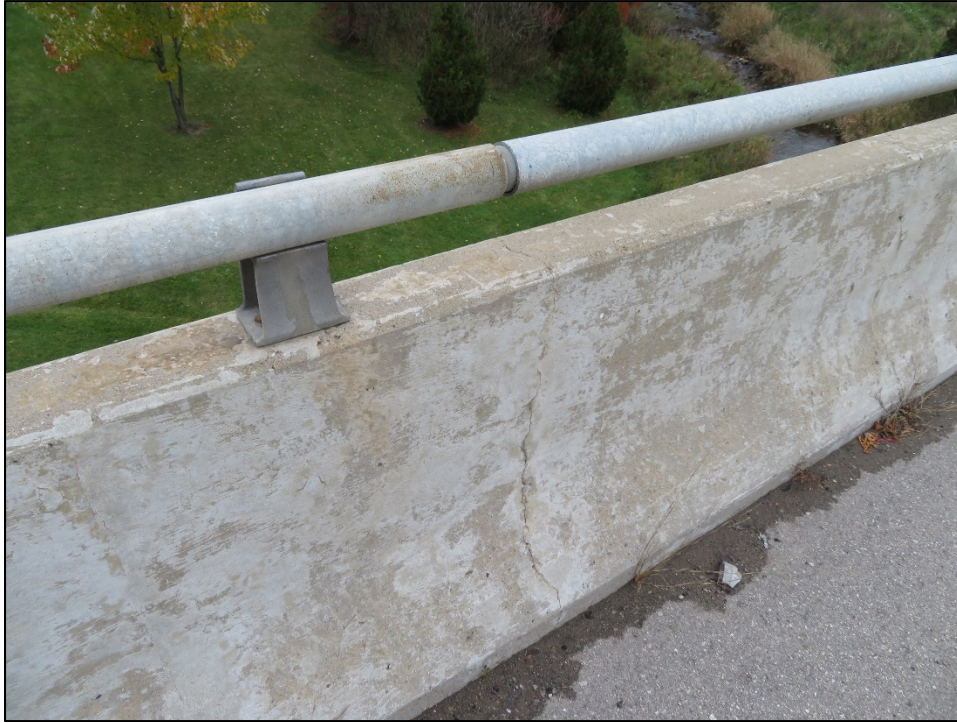
Photo P19 – Typical Condition of North Barrier Wall (fair-to-good condition – cracking)
