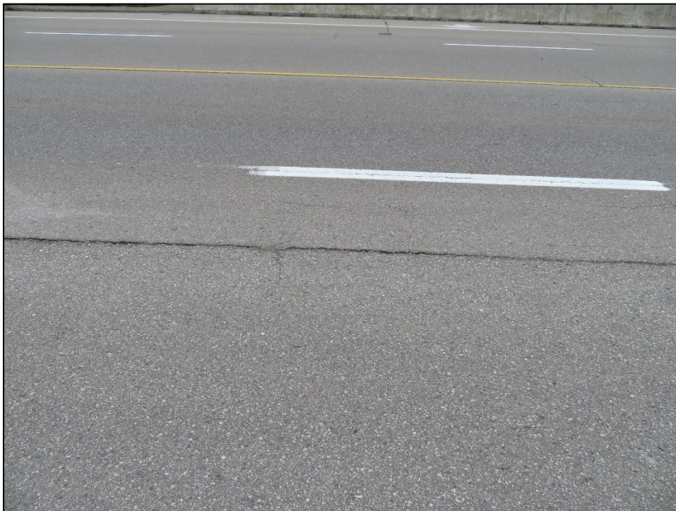
Photo P10 – Typical Condition of Asphalt Riding Surface (fair condition – unsealed cracking)
