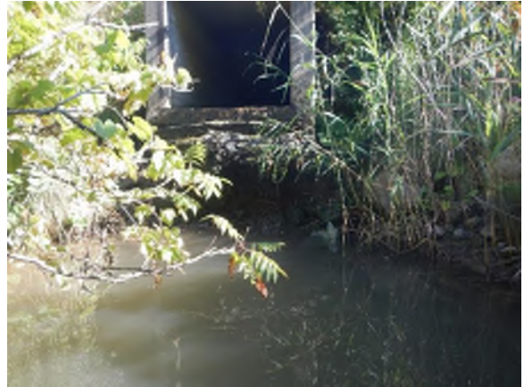
Photo #11: Looking at the downstream end of C1. Culvert is perched due to erosion.
