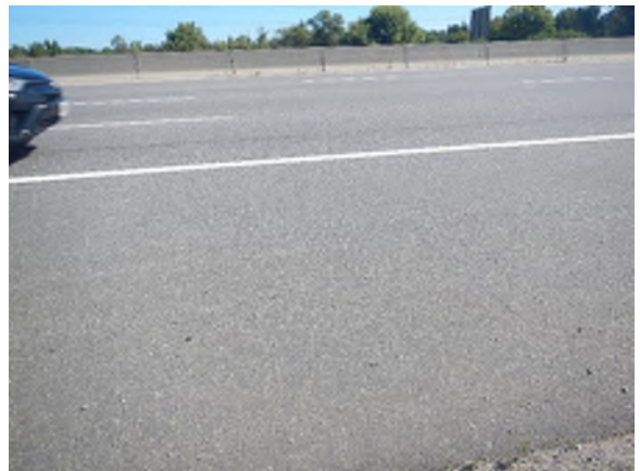
Photo #25: Looking at the condition of the Highway 8 EBL above C4.
