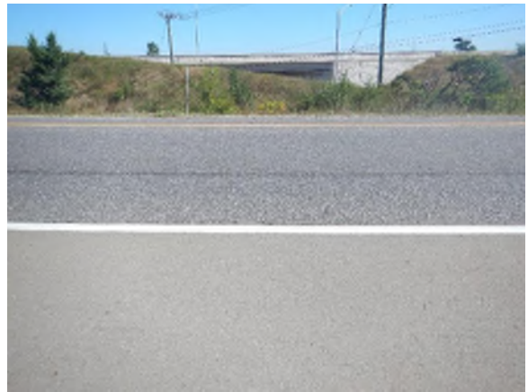
Photo #41: Looking at the road condition above C6.
