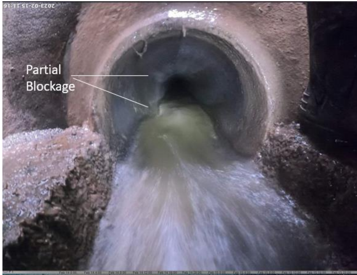
Figure 3-4. Downstream Restriction Observed at WMH71
