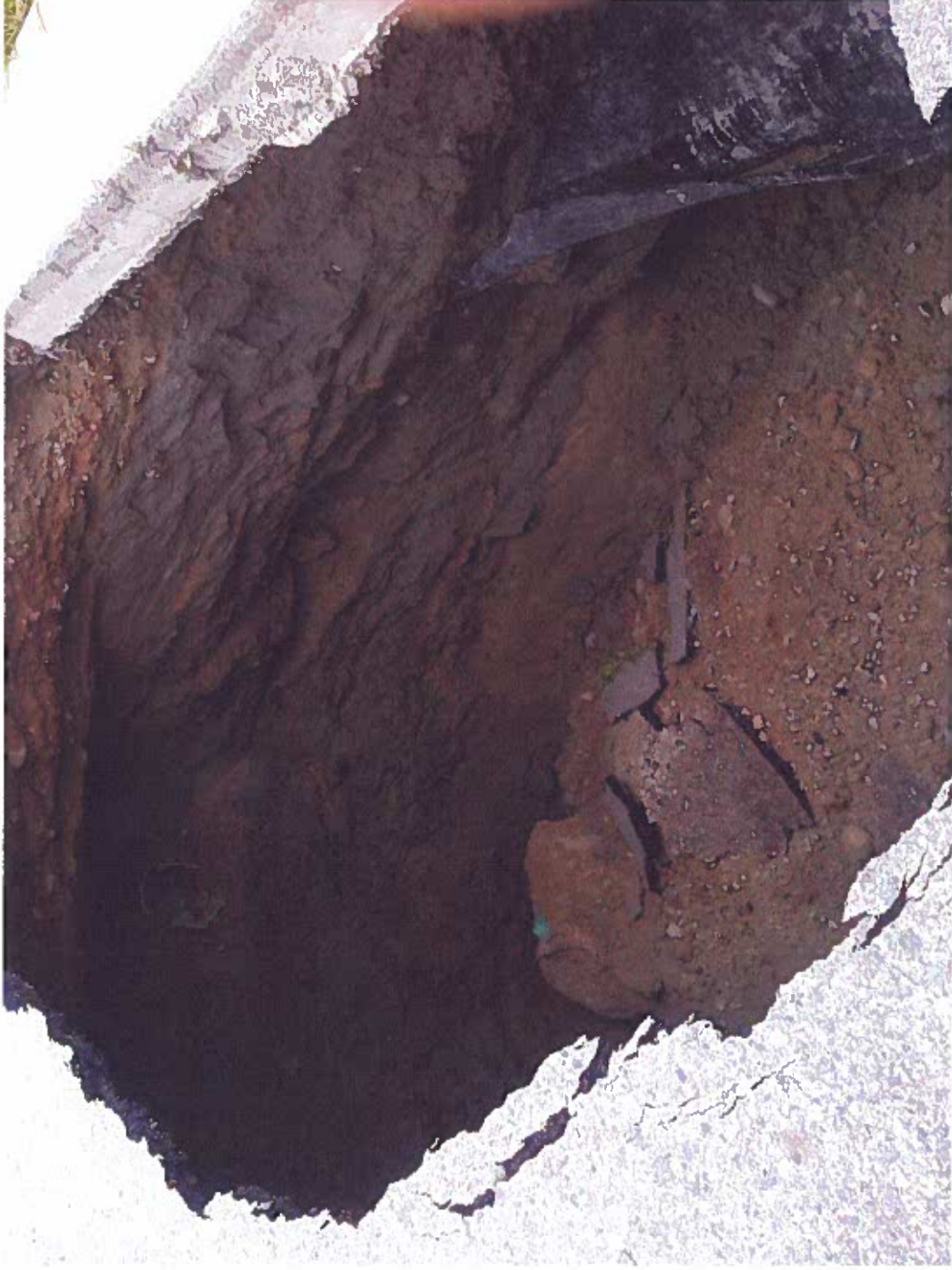
Photo 1. Sinkhole enlarged below asphalt, fabric surround of interceptor drain (near right bottom corner) and broken sanitary sewer (near top centre).
