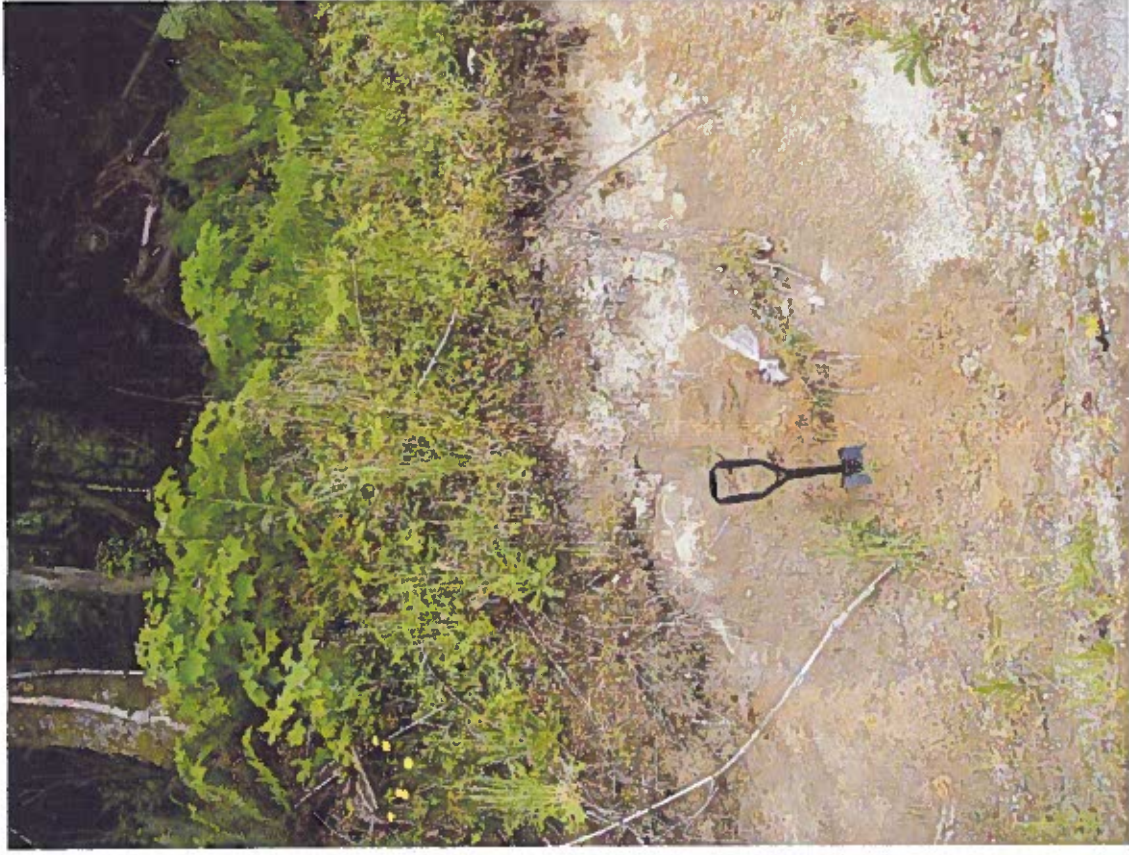
Photo 9. Soil exposure in cut slope opposite Lot 17 (Sta. 3+40, L-200) and sample Sa-6 collection location.
