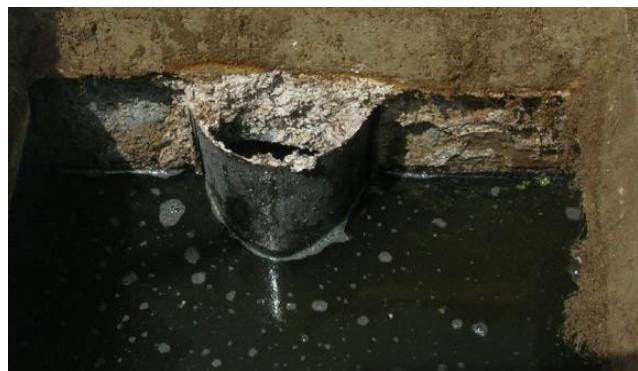
Photo 1 Concrete Corrosion around Outlet Baffle
