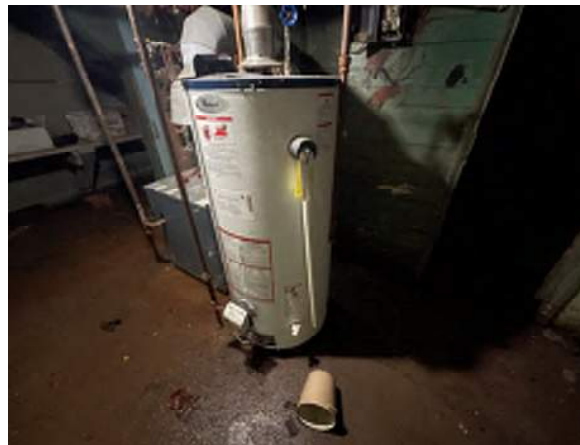
Photo 2: View of the natural gas fired furnace and hot water tank located in the basement of the residential building.
