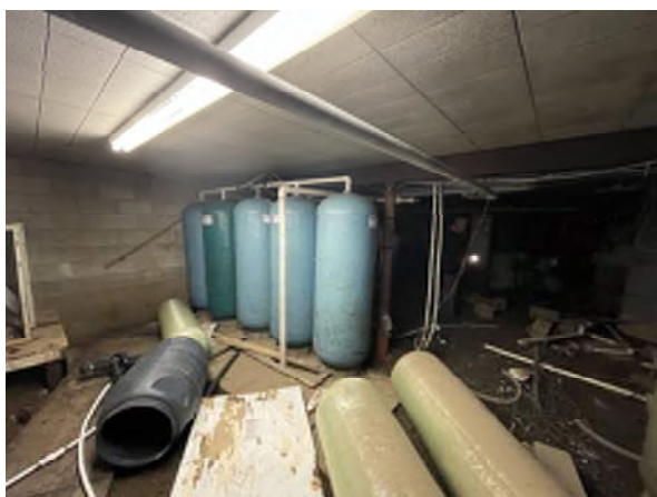
Photo 15: View of the potable water filters, located in the basement of the motel.
