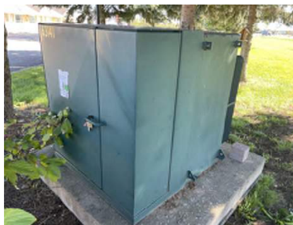
Photo 22: View of the pad-mounted transformer located northeast of the residential building.
