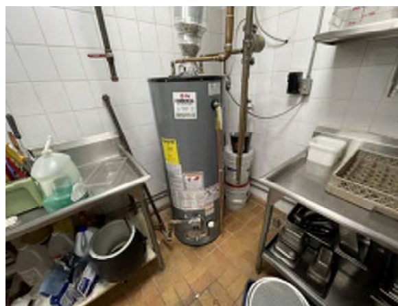
Photo 10: View of the hot water tank located in the kitchen of the nightclub.
