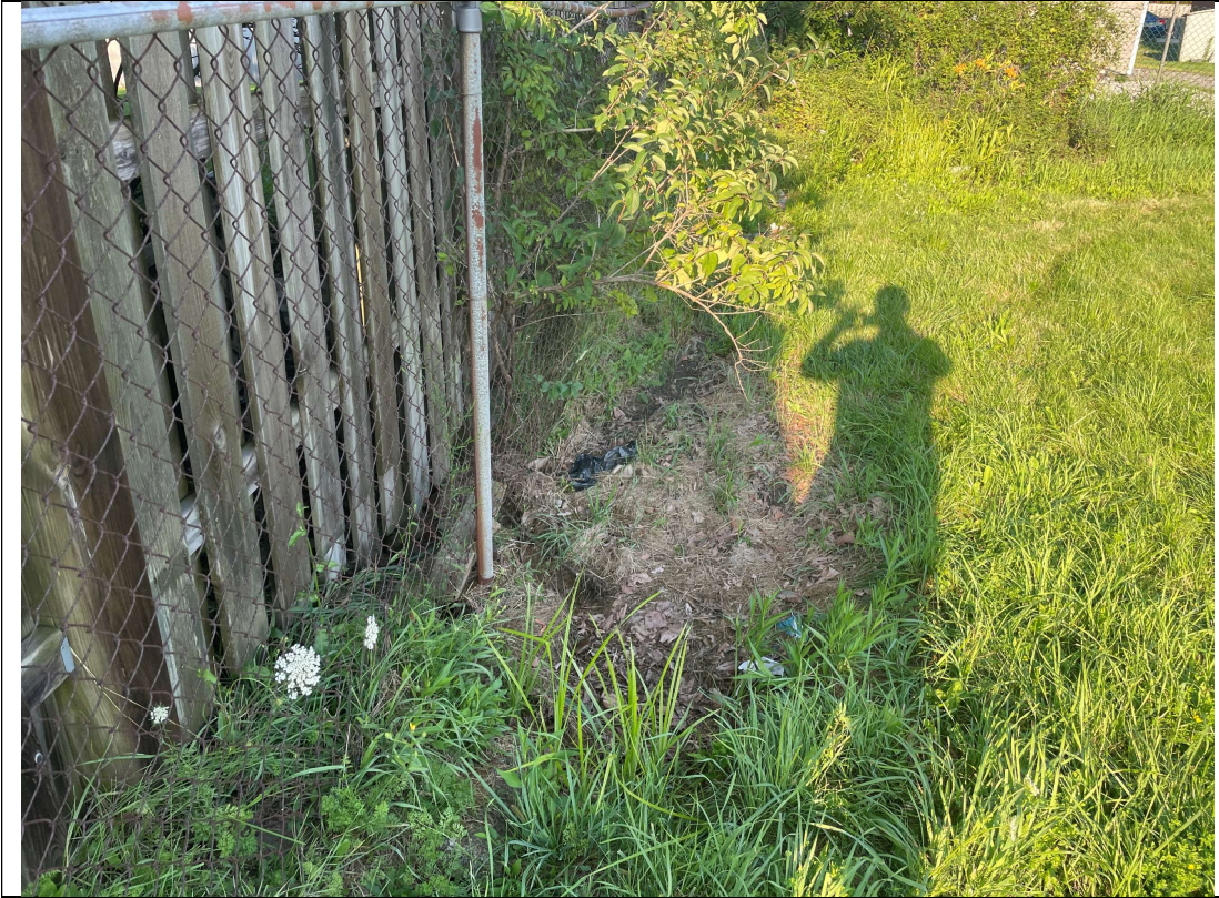
Photo 1: Existing Low Area Near CB Inlet
